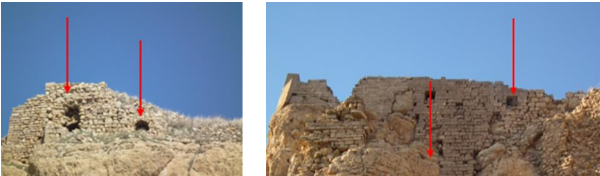
Figure 6. Soil, Debris, etc. in the Masonry. Architectural Gaps Closed with Fillers [2]
