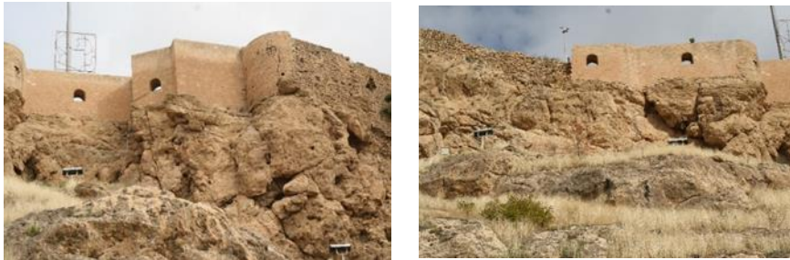
Figure 1. Erosion of the natural rocks on which the walls sit [2]
