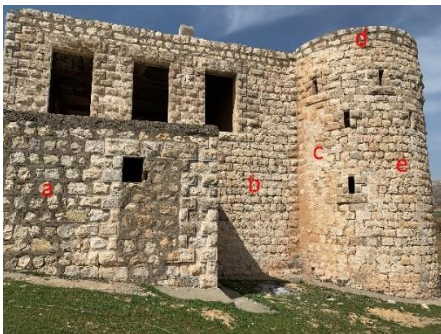
Cement Usage(a,c,d), Surface Loss(b), Surface Loss(c), Joint Discharge(e)
