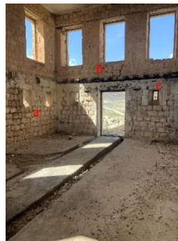
Joint discharge (a), Surface loss (b), Incorrect paint application (c)
