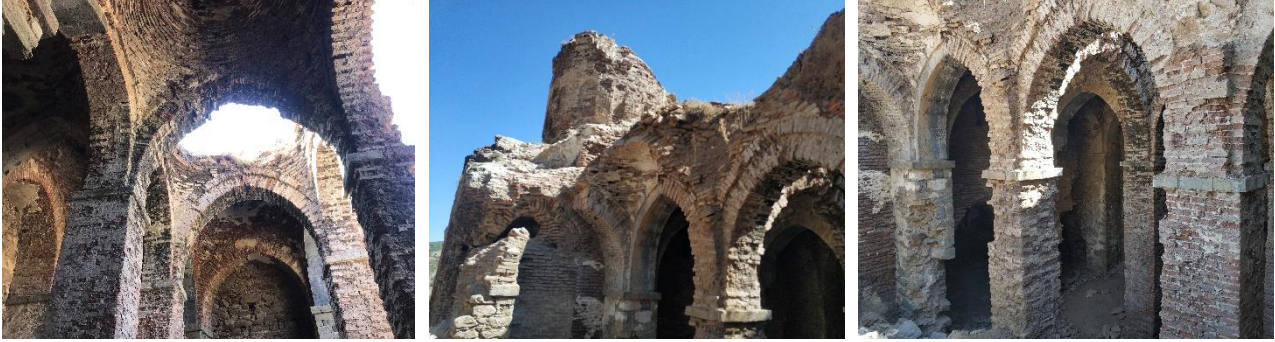
Figure 4. Damaged domes, arches and columns (photo by author)
