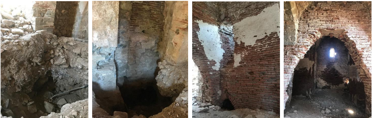
Figure 3. Pits in the ground and damaged walls (photo by author)
